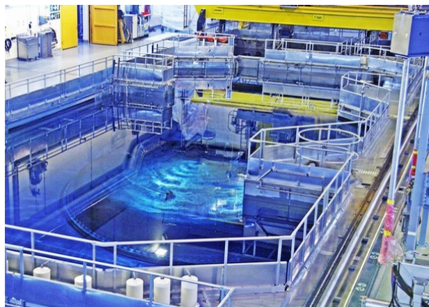
Inside the Forsmark reactor, Sweden
