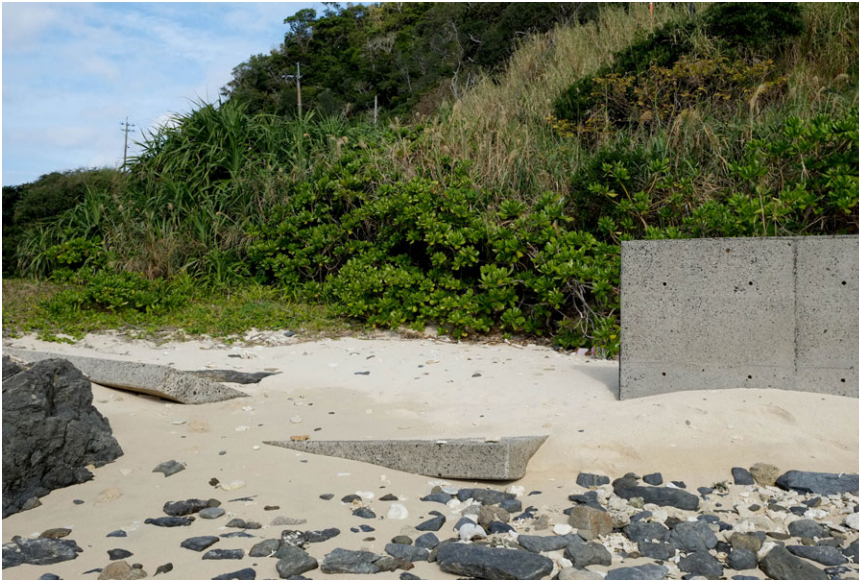
Figure 10: A collapsed seawall on Uttabaru Beach in north Amami. Photo: Charlotte Linton.
